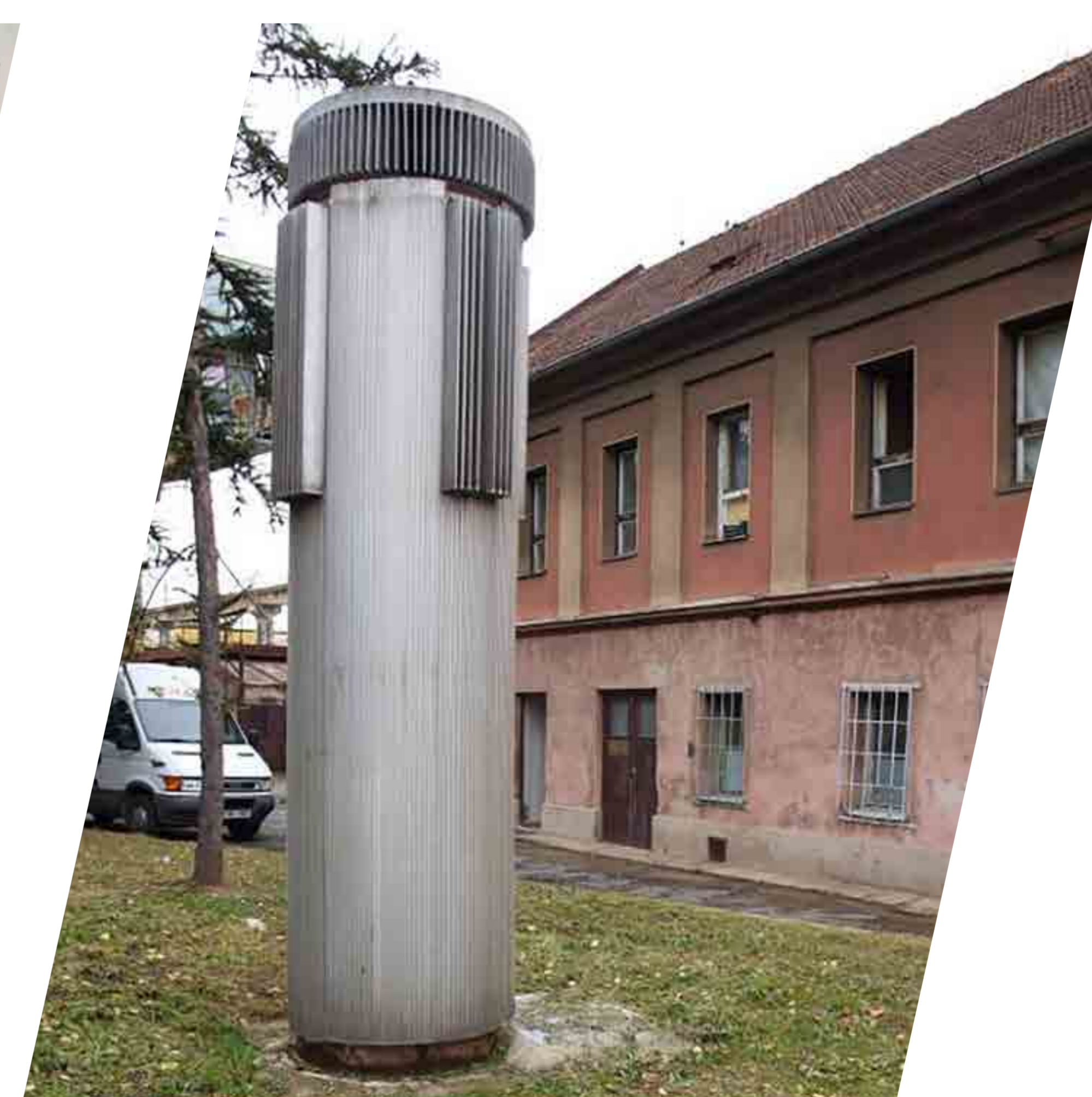
Exhaust and access hole from the VHV power duct.
